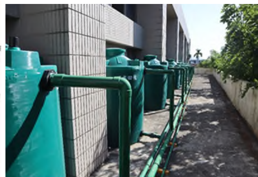
Example of Miaoli Hegang Junior High School Rainwater Storage and Utilization System
