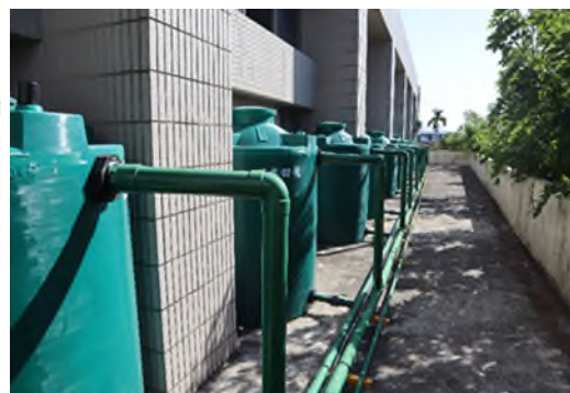
Example of Miaoli Hegang Junior High School Rainwater Storage and Utilization System
