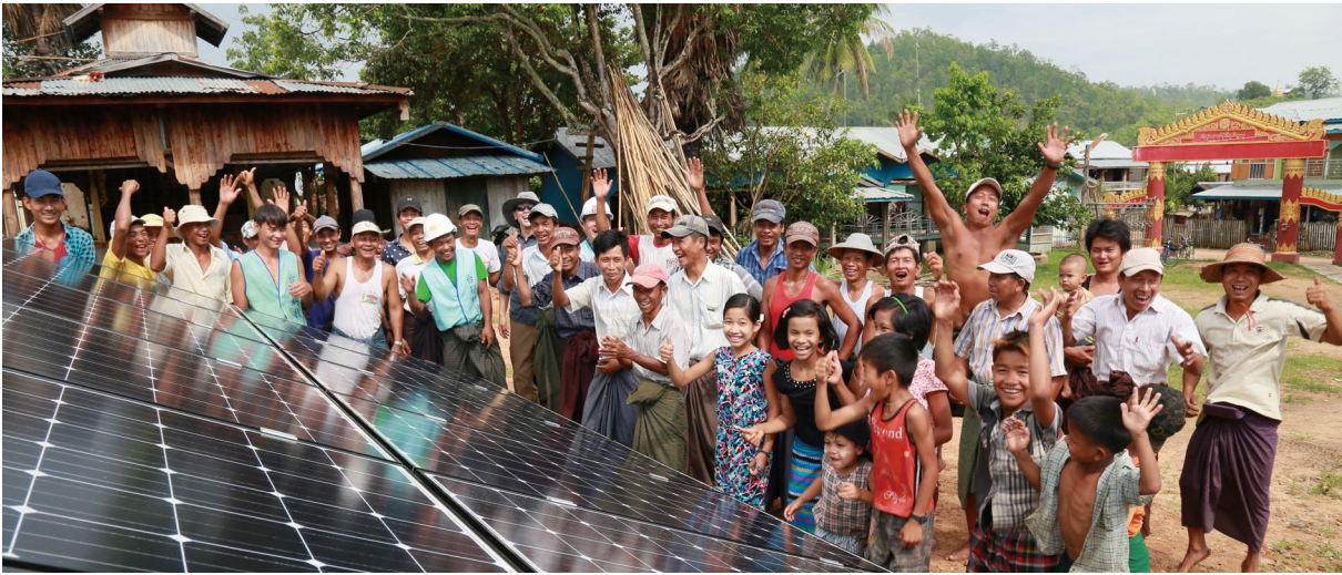
Figure 7.2.1-3: The “Solar PV Mini-Grid System for Lighting in Myanmar Rural Areas” project conducted by the International Cooperation and Development Fund in Myanmar; the villagers and the work team celebrate the completion of the power supply station
